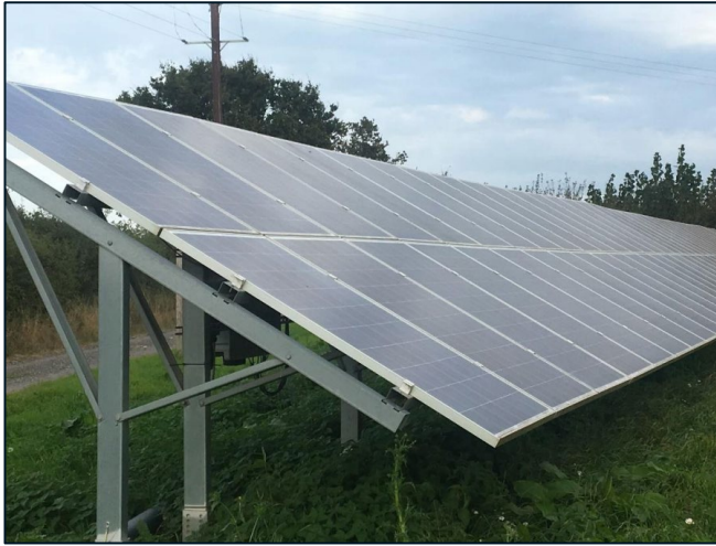
Figure 1-2 Illustrative Array of Solar PV Modules
