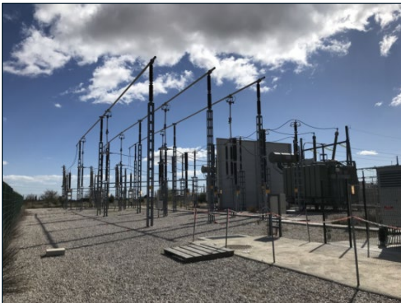
Figure 1-5 Illustrative image of a substation
